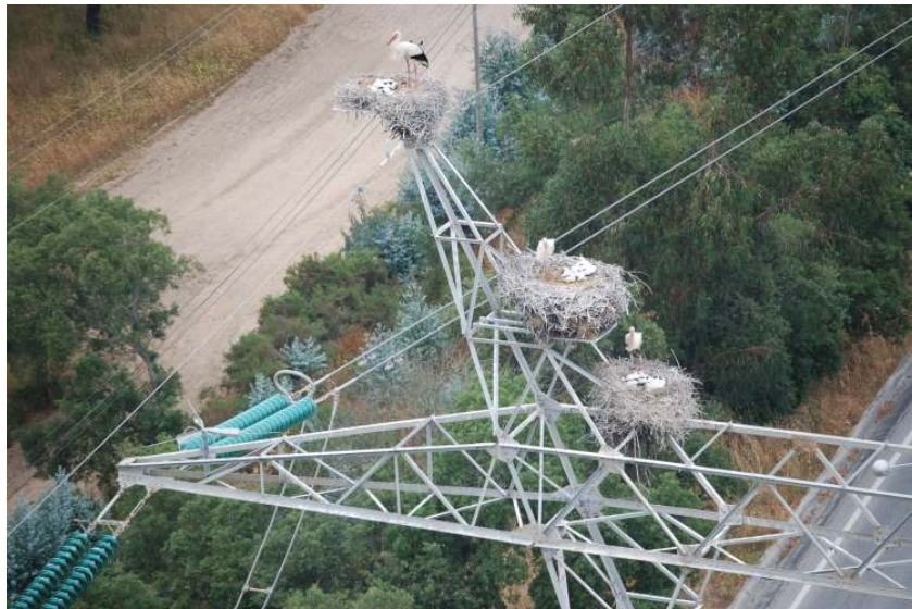
Fig. 5 The two top nests are mounted over platforms on “safe” areas. The bottom one was installed on a hazardous location where droppings affect maintenance work. Notice that near the insulator the horizontal mill deters storks from nesting and standing near the insulator chains.
